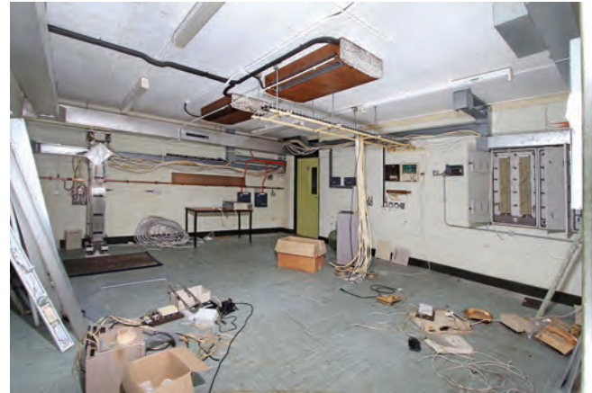
The BT equipment room. The wall cabinet on the right was connected to the Mitel SX2000S ECN cabinet
